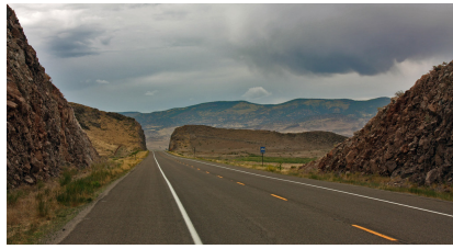
Figure 17.42.: A road cut through a hillside is built by dynamiting the rock along a straight path and removing it, leaving a level surface for pavement.
